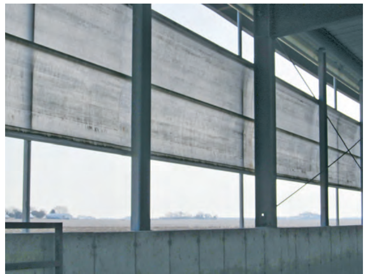
Partially closed curtain
